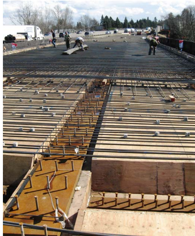
Workers install reinforcing steel (rebar) in preparation for pouring the concrete deck of the new bridge for the Columbia Blvd. on-ramp for southbound I-5 traffic
